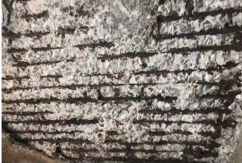
Rusting and peeling areas (front plate)
