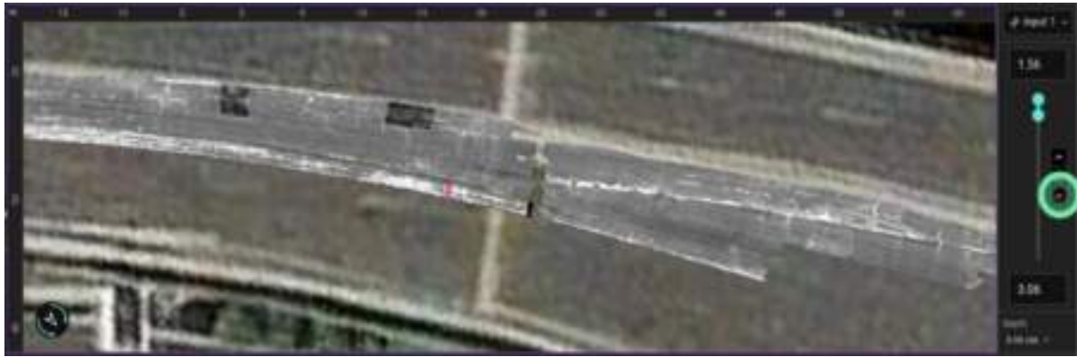
Figure 5. Major surface defects at asphalt layer (cracks)
