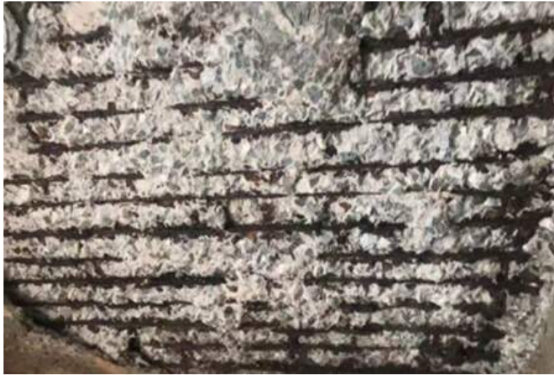
Rusting and peeling areas (front plate)
