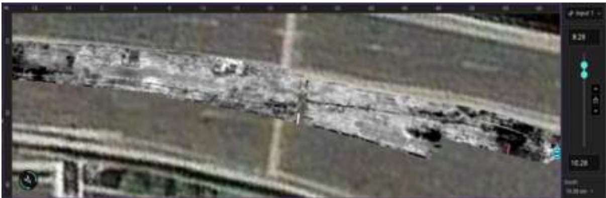
Figure 7. Interface defects between Asphalt-to-Concrete (A/C) layers (Delamination.)
