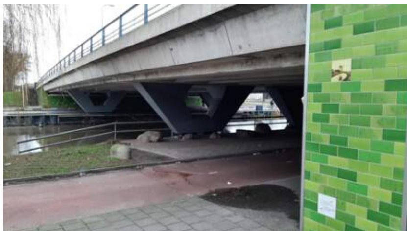
Side view of the bridge and drawings with indications of GPR data collection
